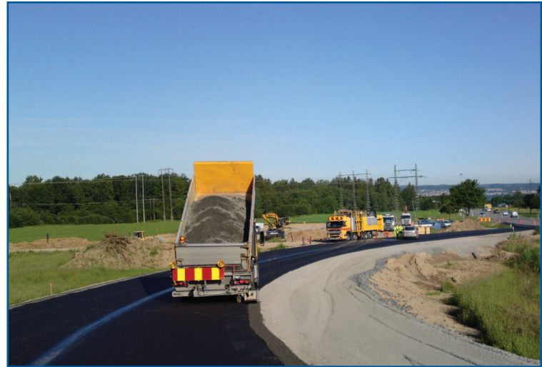
Project Jära Gård, close to Jönköping in Sweden, comprised of the construction of a new in-situ concrete bridge that created a grade separated junction.
